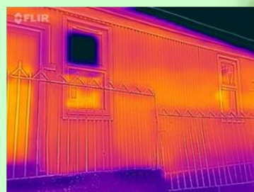
St Barnabas' showing heat loss through the doors and metal walls
