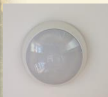
Glass ceiling lights in the toilets
